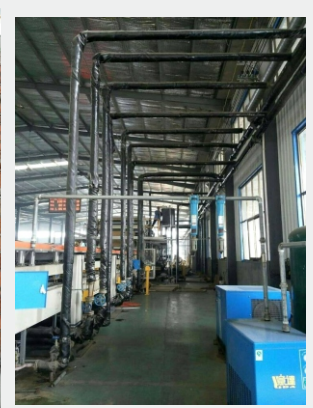
ZQ steam system
